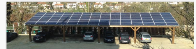
Photovoltaic parking shade area
