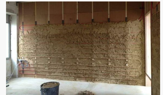
"Low-tech" heating wall in "DUO TERRE" (wooden structure + wood fibre insulation + earth coating)
