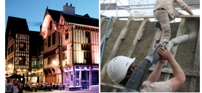
Renovation of Troyes tourist office (10), XVI century. The hemp concrete used to fill wooden frames (30 cm) and the insulation of the roof present both a heritage and hygrothermal interest. An operation based on local know-how, reproducible for the renovation of old buildings in the city center of Troyes.
